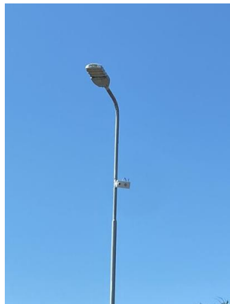
Figure 2: Traffic load sensor on a lighting pole
